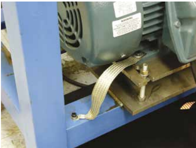
Motor frame bonded to its support by a high frequency grounding strap
